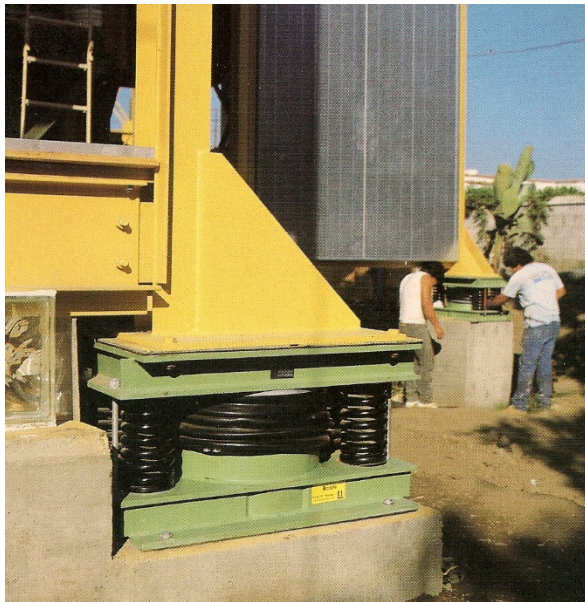
Figure 3. Three story building on springs in North Carolina to dampen the effect of earthquake waves. (Shustov, 1999)
