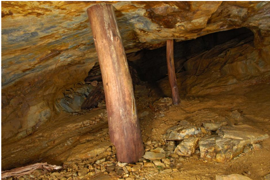
Pit props supporting a stope in the old Hannan’s gold mine in Kalgoorlie
