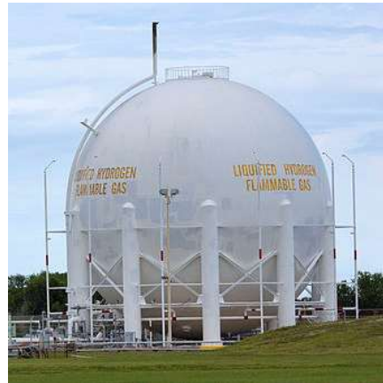
This liquid hydrogen storage tank at Kennedy Space Center was used to fuel the space shuttle. (TomFawls 2013, Creative Commons 3.0)
