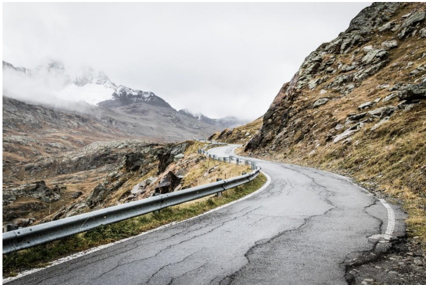
Figure 7. Steep road cutting along a mountain path.
